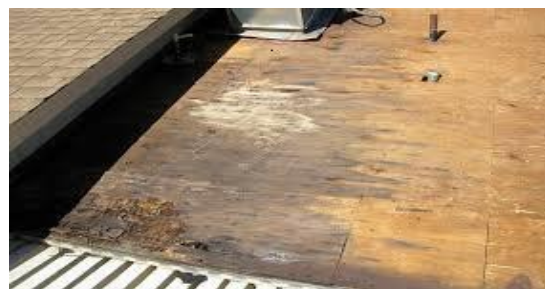
water damaged plywood
